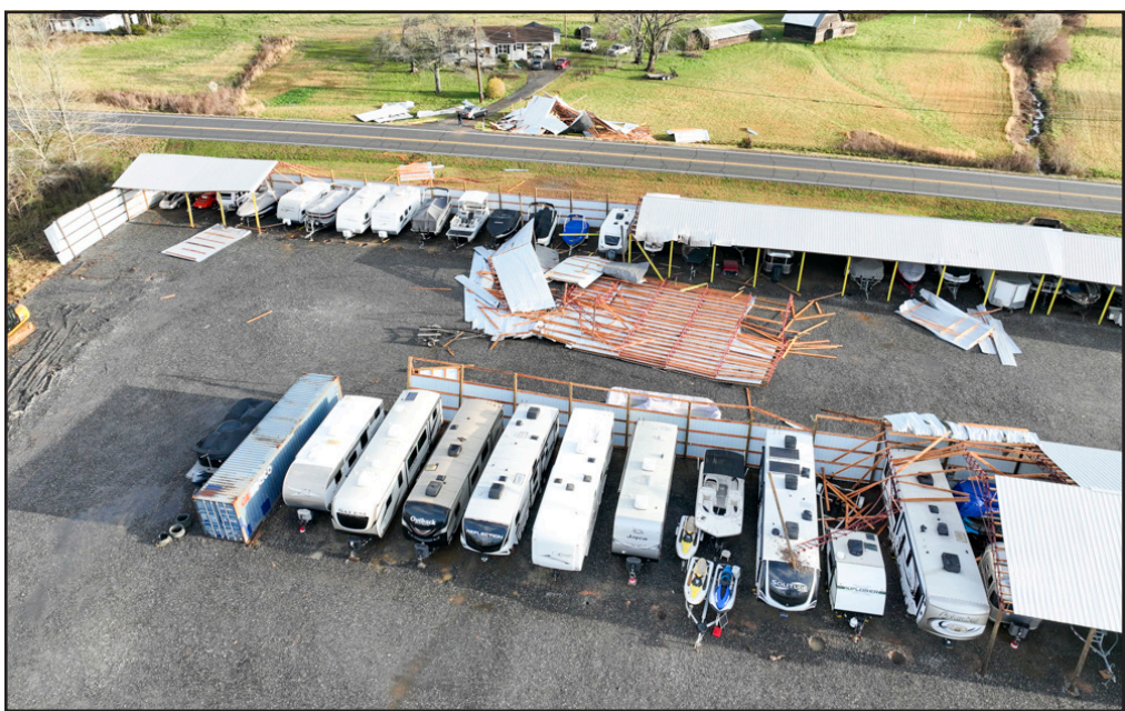
EZ Store It on Lower Bell Creek Road received major damage in the storm over the weekend, but the Phillips Family business owners are just happy nobody got hurt.
